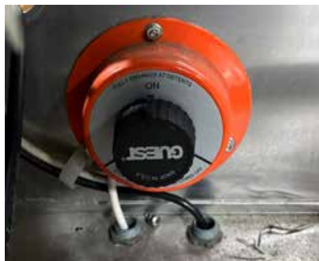
Figure 4 Battery Disconnect Switch
