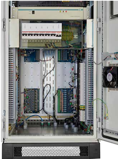
Figure 52 Main Distribution Frame (MDF)
