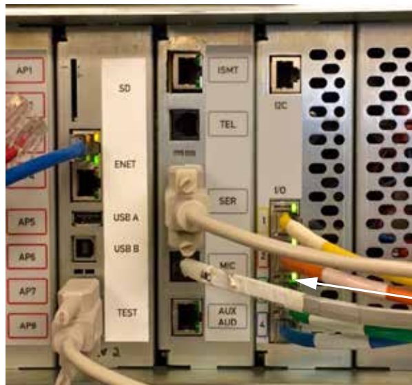
I/O Interface Card 4 x RJ45 Cables (RS485 Serial)
